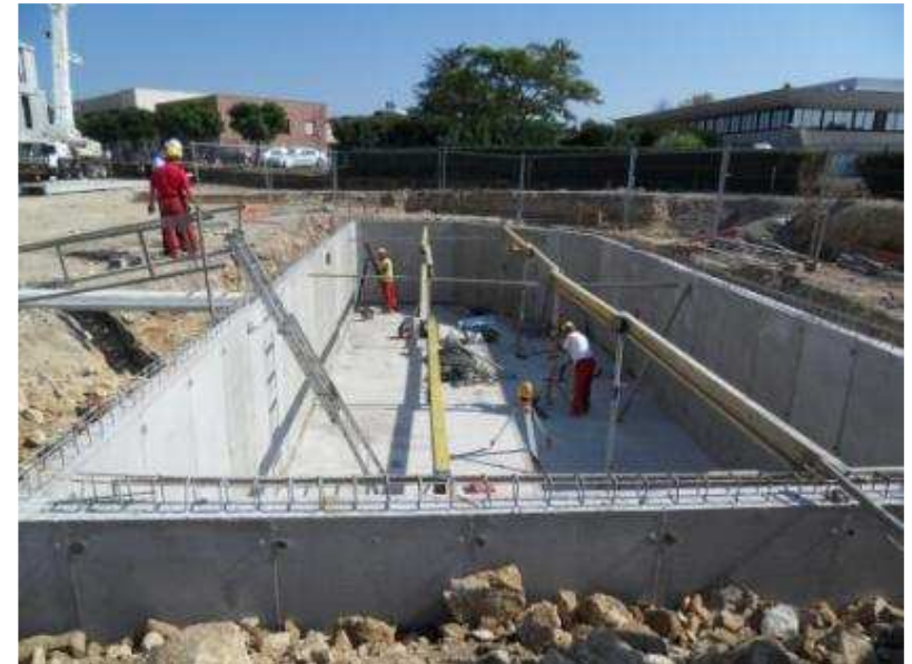
MAAF Assurances, Chauray (79) – cuve de 160 m 3
